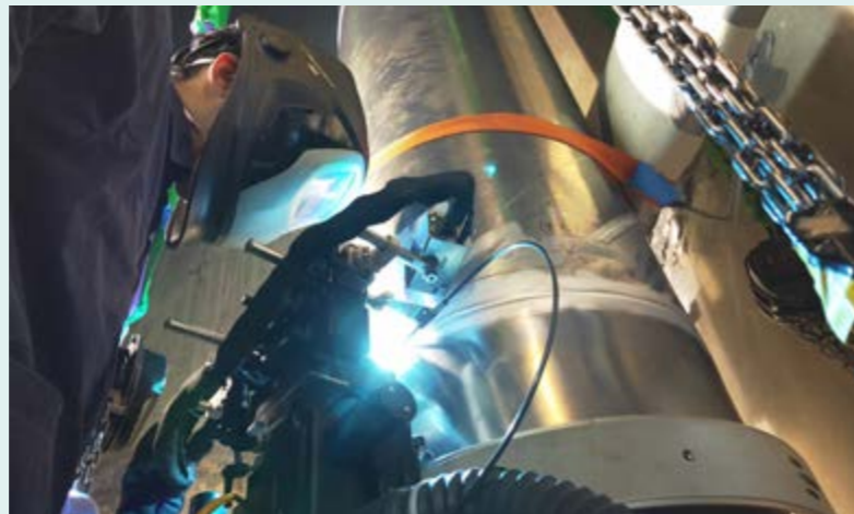
GIL maintenance site of Xiluodu HPP left-bank
